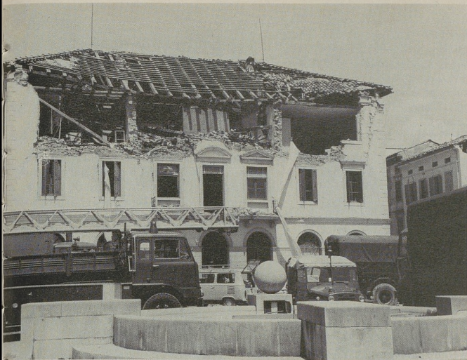
At Buia, Italy, the quake took 42 lives. This is the city hall.
