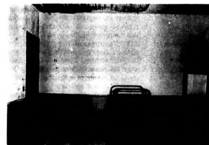
Room on third floor Administration Building. Now condemned and closed. Formerly used as girls dorm room.
