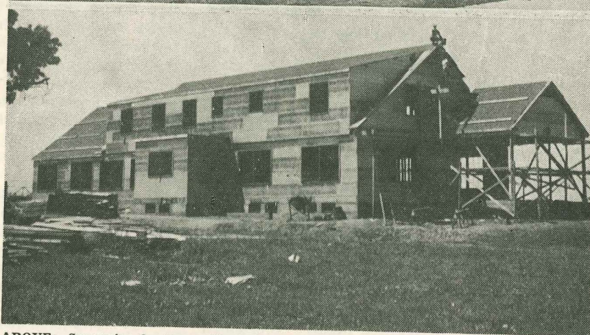
ABOVE: Surveying for the auditorium and gymnasium at the Kentucky Baptist Children's Home, Glendale, Ky. The foundation is already laid. BELOW: Shaping up the girls' Cottage.
