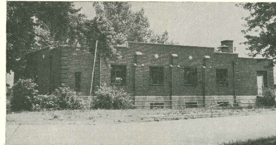
This building is being remodeled to take care of Convalescent patients at the Baptist Home of Northern Kentucky.
