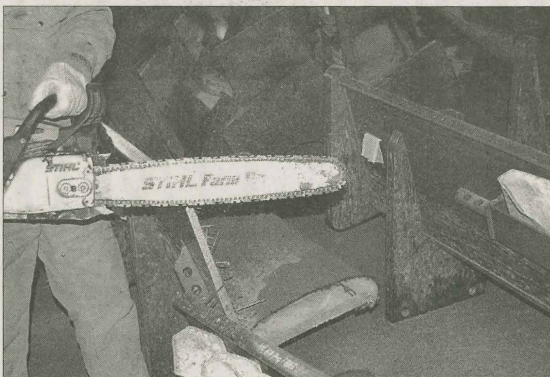
OUT WITH THE OLD Mold-covered pews at First Baptist Church of Chalmette, La., had to be removed with a chainsaw. Members of the church, in the St. Bernard Parish in metro-New Orleans, still don't know when they can rebuild. (BP photo by Keith Manuel)
