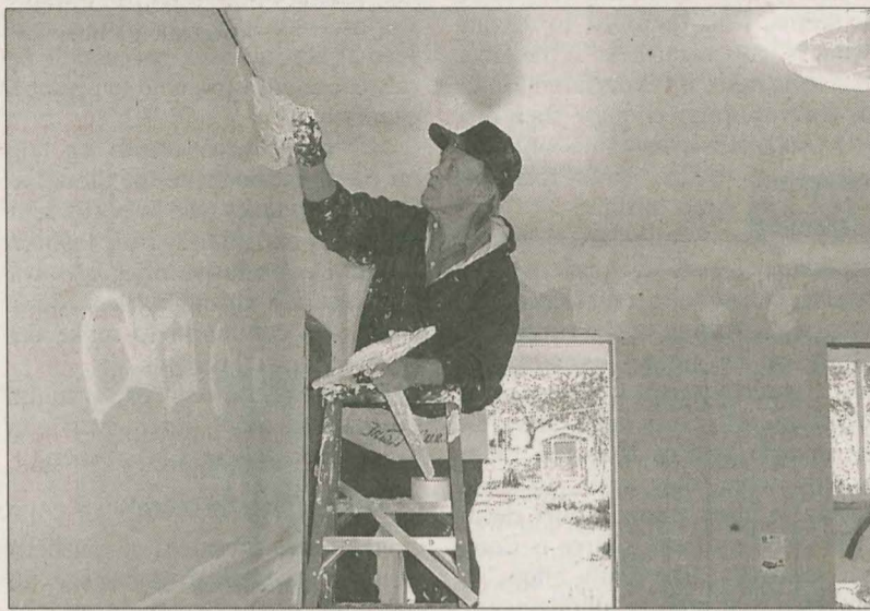
DRYWALL Don Preuit, a member of Main Street Baptist Church in Williamsburg, puts mud on the drywall of a home in Pascagoula, Miss. Baptist volunteers have mudded out more than 3,700 homes and repaired more than 1,200 in Jackson County, Miss. (Photo by Vicky Edwards)
