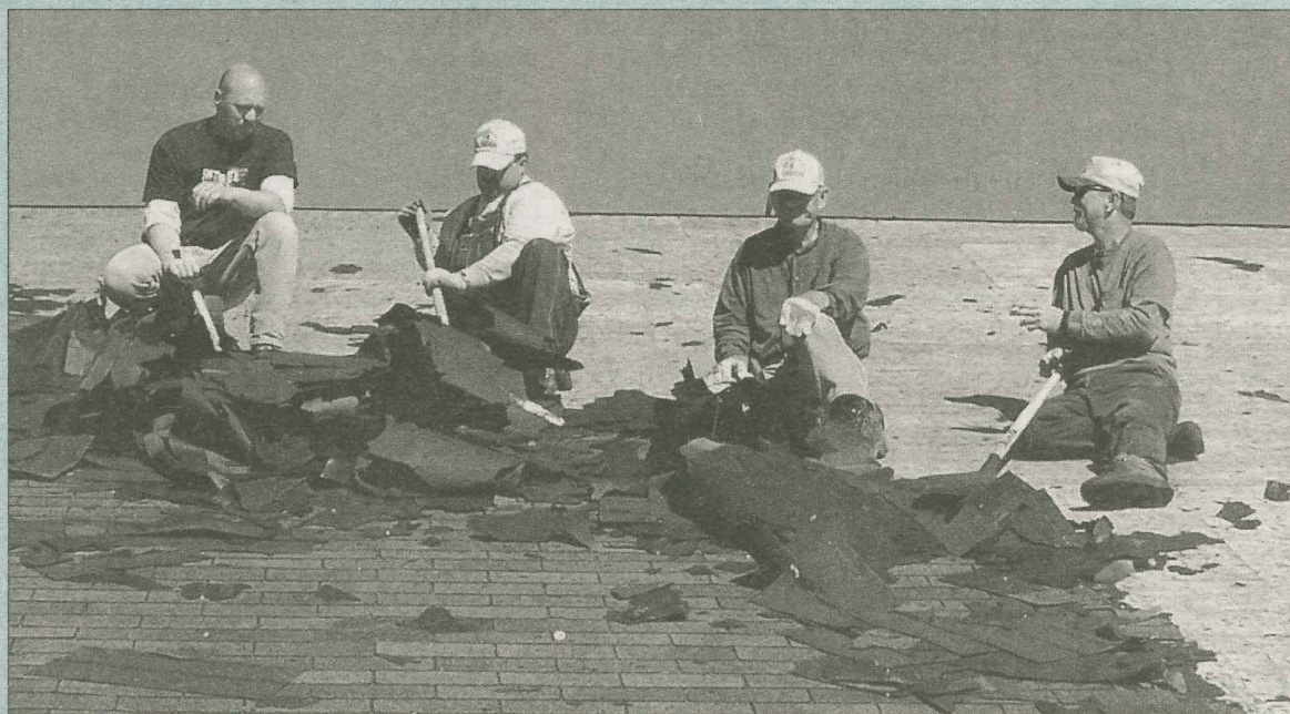
REPAIRING HURRICANE DAMAGE Volunteers from Hazard (from left) Glenn Shields and Carl Collier of Upper Second Creek Baptist Church, Winston Fields of Big Creek Baptist Church and Steve Howard of Upper Second Creek Baptist Church remove damaged shingles from the roof of the Jackson Baptist Association building in Pascagoula, Miss. Three teams from Three Forks Baptist Association in Hazard have traveled to the Gulf Coast this winter. (Photo by Cordis Bishop)
