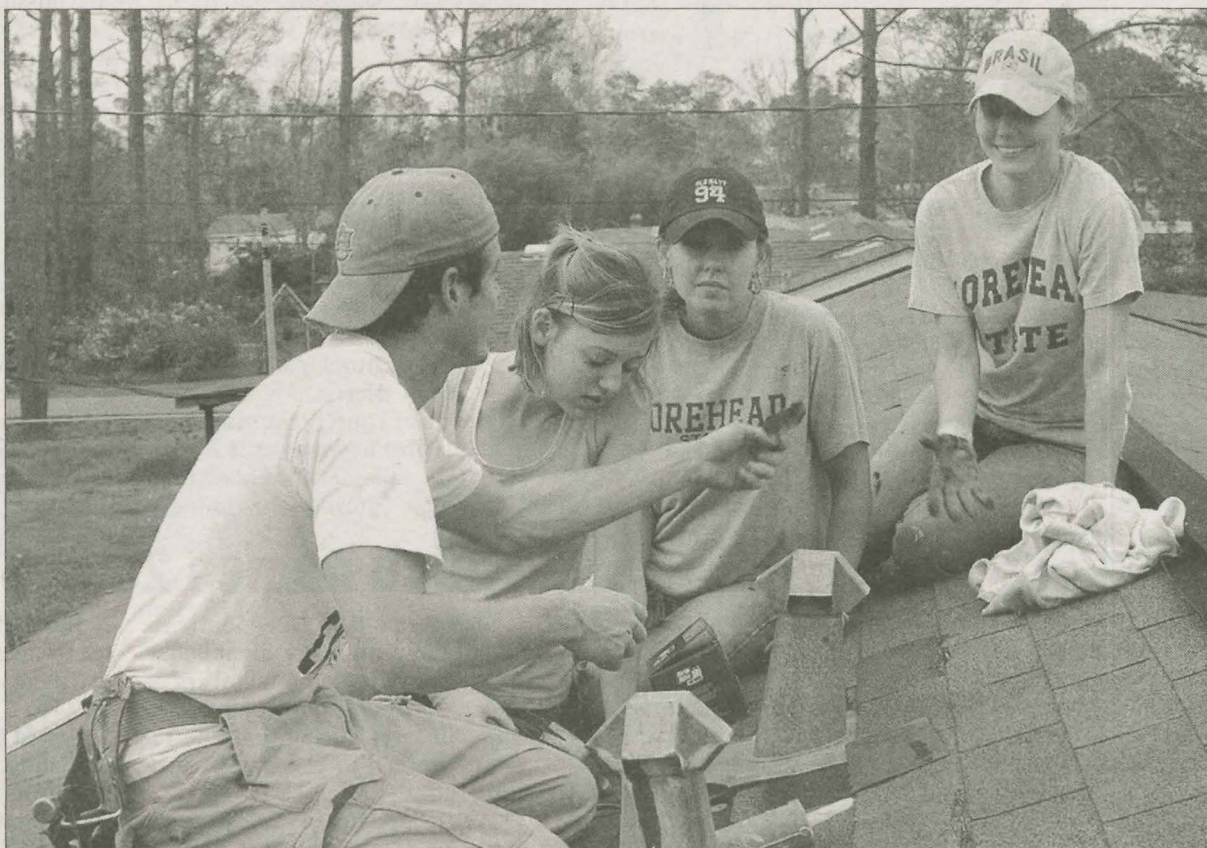
ROOF REPAIR Morehead State Baptist Collegiate Ministry students Doug Kline (from left) and Megan Maraz work with fellow students Nikki Pergram and Sarah Fischer in Gulfport, Miss. (Morehead State University photos)
