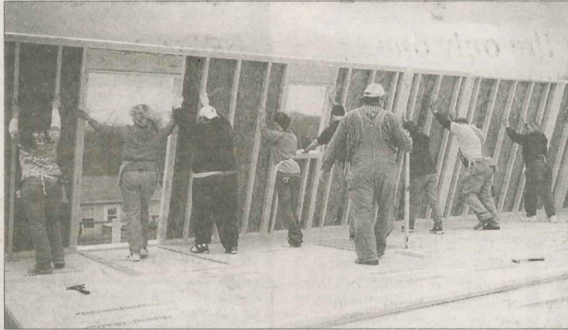
RAISE THE WALLS Volunteers put an exterior wall in place during the Kentucky Changers Blitz Build in Morehead, March 8-18. Volunteers from four colleges took part in the effort. (Photos by Elaine Koch)
