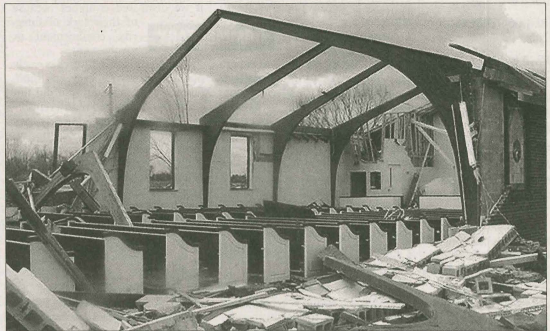
DESTROYED The sanctuary of Sinking Fork Baptist Church in Christian County was hit by an F-3 tornado.
