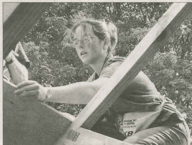
HABITAT HOME Allyson Snellin a member of Locust Grove Baptist Church in Locust Grove, Ohio, works atop the roof of a Habitat for Humanity house in Russellville.
