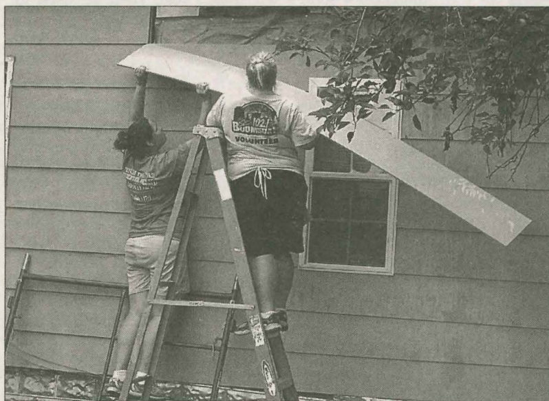
INSTALLING SIDING University of the Cumberlands students Sarah Whitaker and Tracy Smith install siding outside a newly renovated home. The home renovation is one of several projects to be completed by Mountain Outreach this summer.
