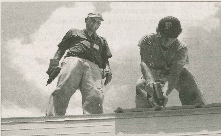
ROOF WORK Lawrence Bolin (left) of King's Mountain, N.C., watches Kary Ballew of Fairfield, Texas, install roofing on a carport. Volunteers worked on 21 homes during the weeklong ministry effort.
