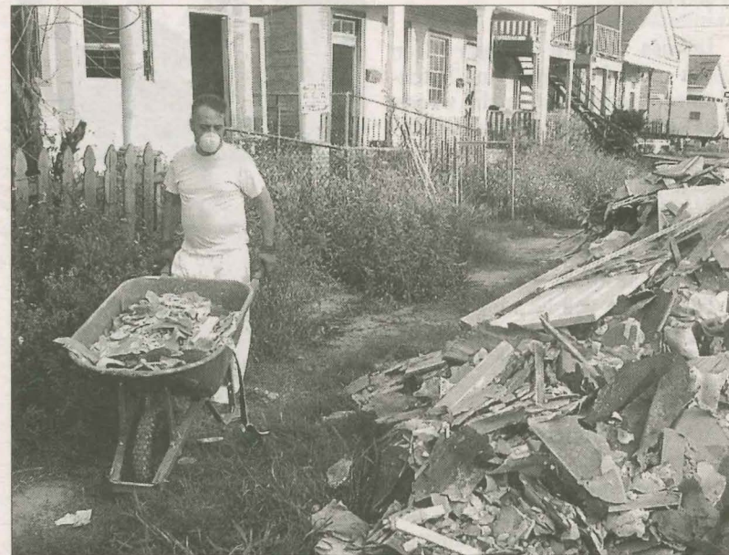
CLEANUP CONTINUES Don Sweet, a member of Porter Memorial Baptist Church in Lexington, carries rubble from a house in an area of New Orleans hard hit by Hurricane Katrina. He and other volunteers from Porter Memorial traveled to "The Big Easy" last month. (© Lexington Herald-Leader photos by Frank Lockwood)
