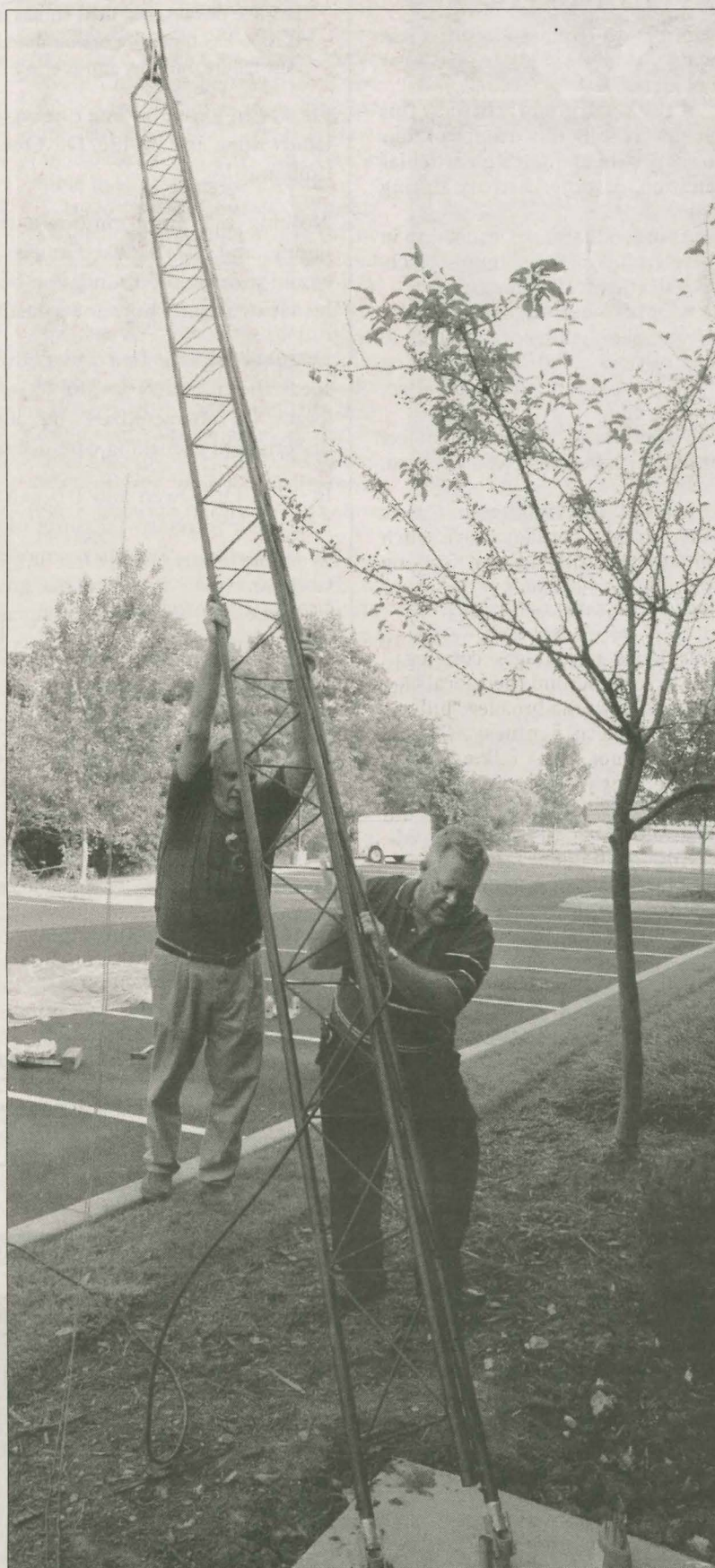
PLANTING ANTENNA Tom Westerfield (left), a disaster relief volunteer from First Baptist Church of Hopkinsville, and Larry Koch, director of Kentucky Baptist disaster relief, install an antenna outside the Baptist building in Louisville. A new amateur radio station will help coordinate disaster relief work around the country where phone lines and cell towers have been disabled. (KBC photo by Robert Reeves)
