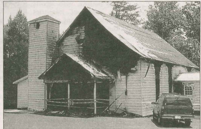
CHURCH FIRE Concord Baptist Church in Monticello was underinsured when an electrical fire destroyed the church facility in July.
