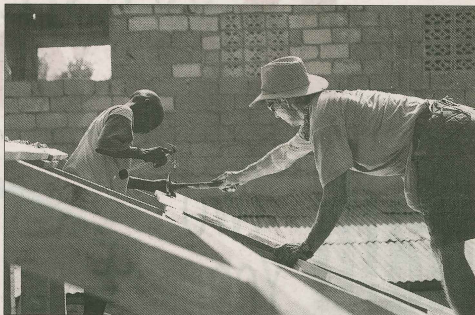
HOME SWEET HOME A Southern Baptist volunteer (right) and a Haitian worker build a new house for earthquake survivors in Port-au-Prince, Haiti, as part of the Rebuild Haiti relief project. Since the 7.0 earthquake rocked the island nation on Jan. 12, 2010, Rebuild Haiti has constructed 2,800 houses in 30 hard-hit communities. (BGR photo)
