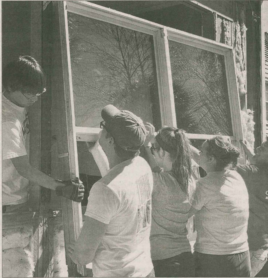
SPRING BREAK MISSIONS A team of Campbellsville University students work to remove a window from a damaged home in New Orleans. (Photo by Sarah Creason/CU)
