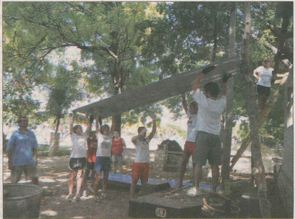
MANUAL LABOR Students from Main Street Baptist Church in Williamsburg install a roof on the generator house at Camp Le Phare as part of their mission trip with Crossings in Haiti. Chris Leib (far left), who directs Camp Le Phare and is an employee of Baptist Haiti Mission, supervises the work. (Photos courtesy of Main Street Baptist Church)
