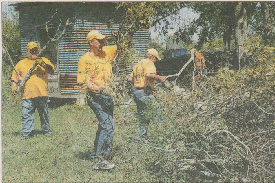
CLEANUP UNDERWAY A Southern Baptist Disaster Relief chainsaw team from Cedar Crest Baptist Church in West Monroe, La., clears debris from a fallen tree at a residence. (Photo by Karen Willoughby/Louisiana Baptist Message)
