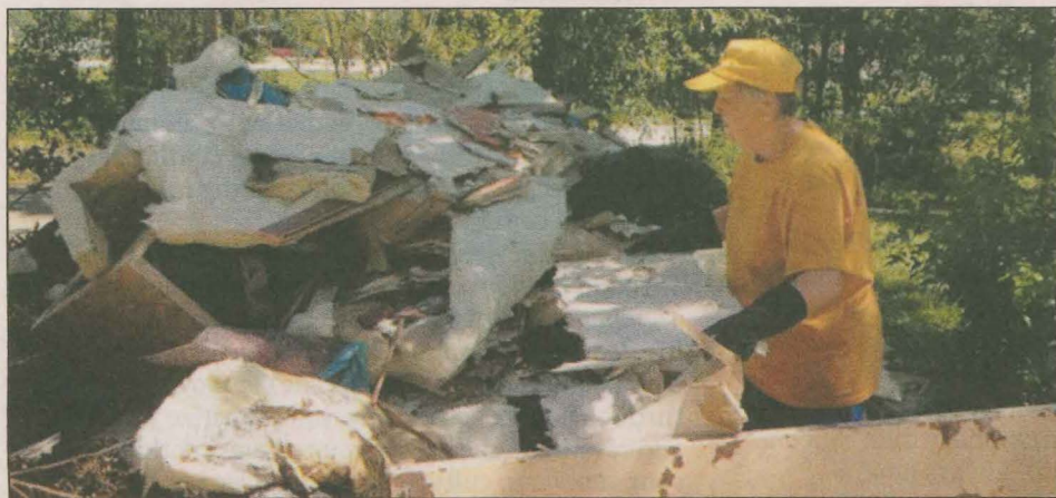
MUD OUT Janice Gaines, of Benton, serves with flood recovery work in Louisiana after Hurricane Isaac. Gaines is a member of Hamlet Missionary Baptist Church.
