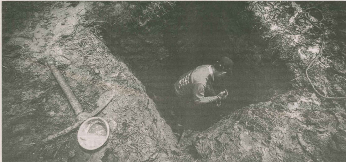
LIFE-SAVING WORK In Mongolia, digging by hand through several meters of rain-sodden dirt and permafrost is the best way to construct simple but effective wells. Lined with wooden walls and void of any moving parts, these low-maintenance wells will provide local herder families with water for many years.
