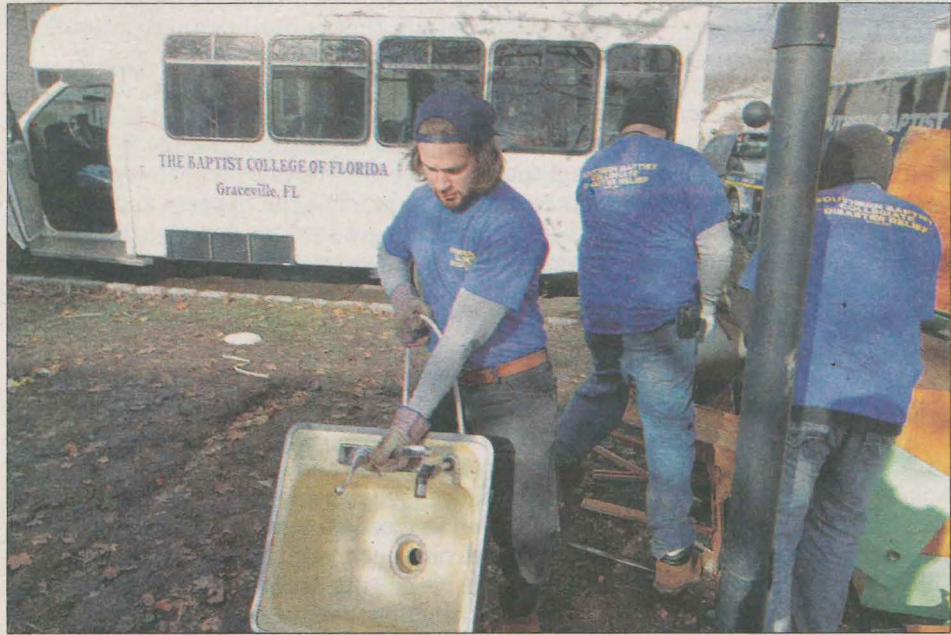
CLEANING UP Jordan Crawford, a student from Florida Baptist College, adds a kitchen sink to a debris pile from a gutted Staten Island home. Crawford was among hundreds of college students volunteering with disaster recovery efforts during their schools' winter breaks. (Photos by Adam Miller/NAMB)
