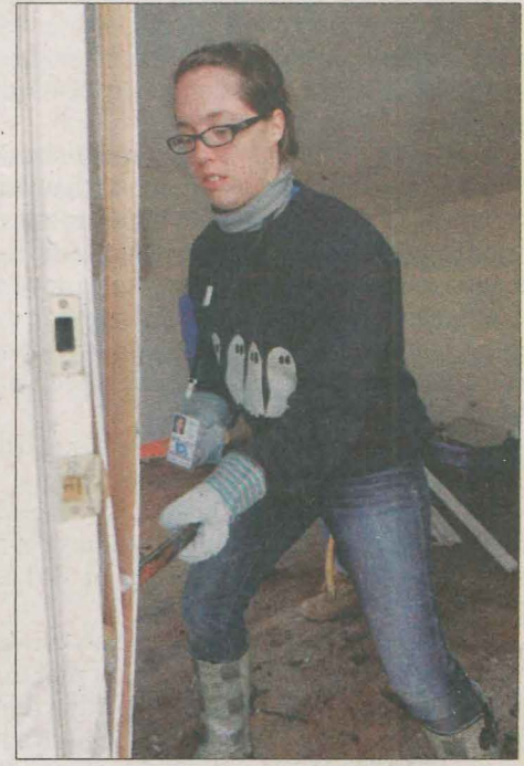
RECOVERY WORK Katie Lilly uses a crowbar to remove molding from a Staten Island home to help the owners prepare for a rebuild of their storm-damaged property.
