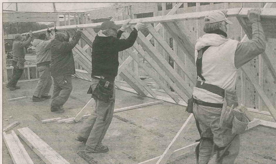
Volunteers from several Kentucky Baptist churches recently worked together to build new houses for victims of the tornado that struck West Liberty last year. (Photo by Larry Brannin/KBC)
