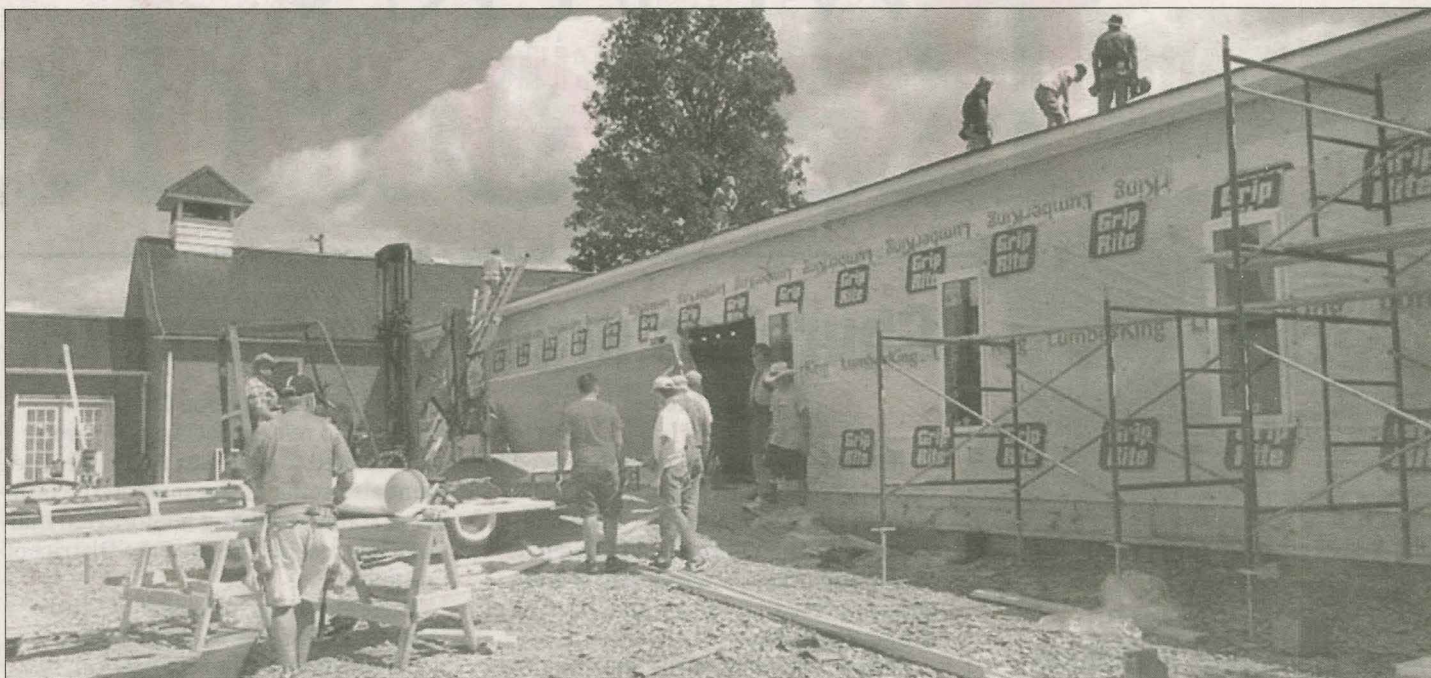
Volunteers with Baptist Church Builders of Texas doubled the size of Polly Ann Baptist Church in Eubank in only seven days. (Photos provided by PABC)
