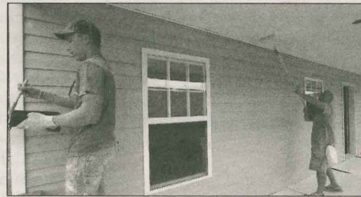
UC student Dirk Berta (left) and Josh Bowman, of Wofford Baptist Church in Williamsburg, paint the porch ceiling of a Mountain Outreach home. (UC)
