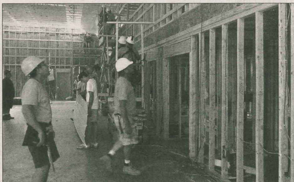
A 126-member team of Carpenters for Christ from Lakeview Baptist Church in Auburn, Ala., work on a multi-purpose building for Salem Baptist Church in Pembroke. The Alabama Baptists were assisted through the Kentucky Baptist Convention's missions mobilization team. (KBC)
